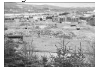
Workers go about in their excavators on Tuesday morning clearing away the final remnants of the former Dr. Charles A. Janeway site in Pleasantville.
